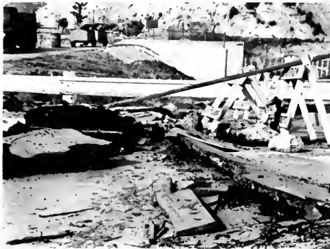
Photo 7. Example of street damage that affected travel to and from residential areas.
